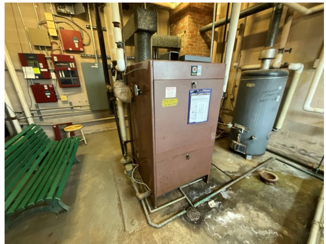
16 - SECOND BOILER ROOM
