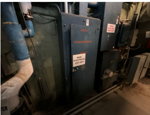
17 - MAIN DISTRIBUTION PANEL
