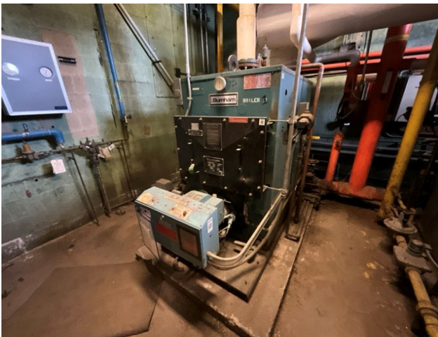
15 - MAIN BOILER ROOM
