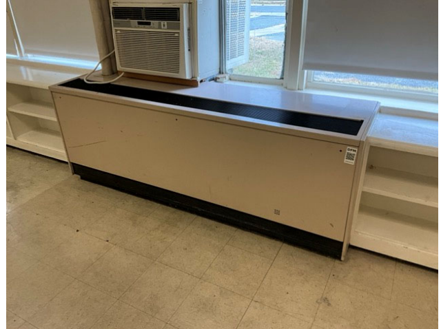
14 - CLASSROOM UNIT VENTILATOR
