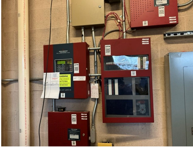
19 - FIRE ALARM PANEL
